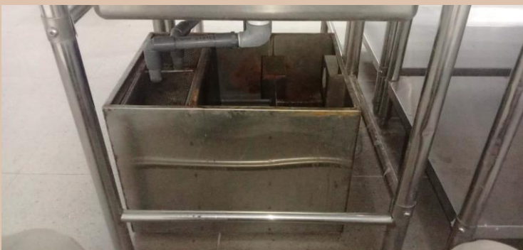
Waste Water Filtering in the Canteen Kitchen
